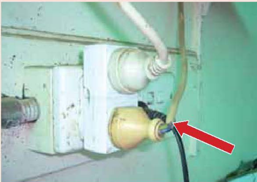
Damaged power leads which have not been inspected and tagged are used.
