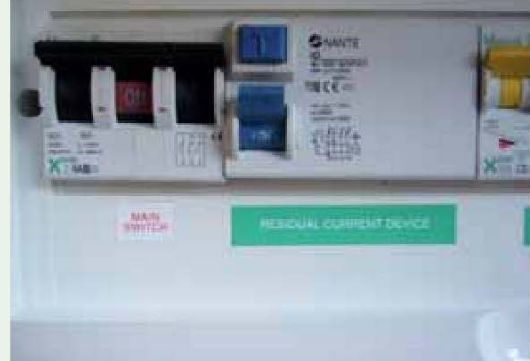
Residual Current Device (safety switches) hard wired into all electrical switch boards.
