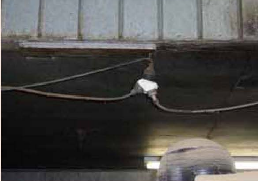
Portable power leads permanently used instead of fixed wiring.
