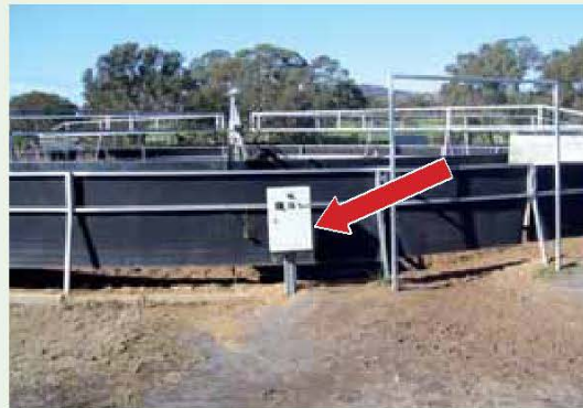
Horse walker controls are located in close proximity to gate and fitted with an emergency stop button.
